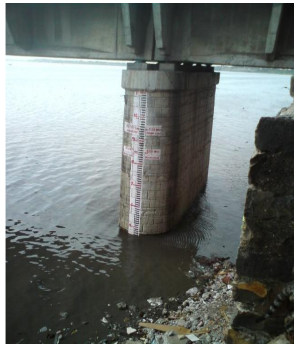
Fig.5. River Gauge Station at Nehru Bridge / Hope Bridge, Surat
